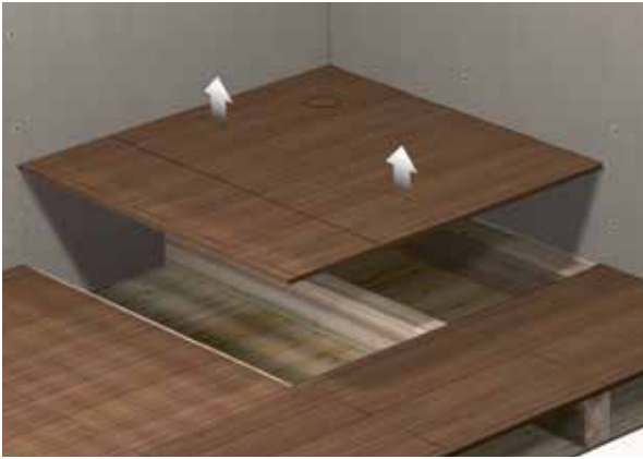
1. Remove floorboards to the nearest joist where the shower tray will be located.
